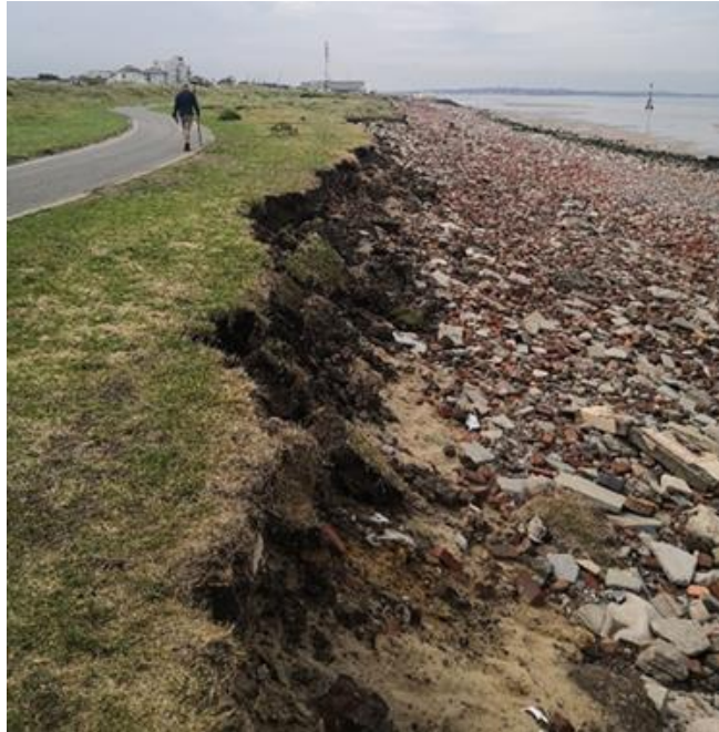
Figure 7: Coastal erosion along the Crosby coastline is posing a risk to a large diameter rising main and pumping station
