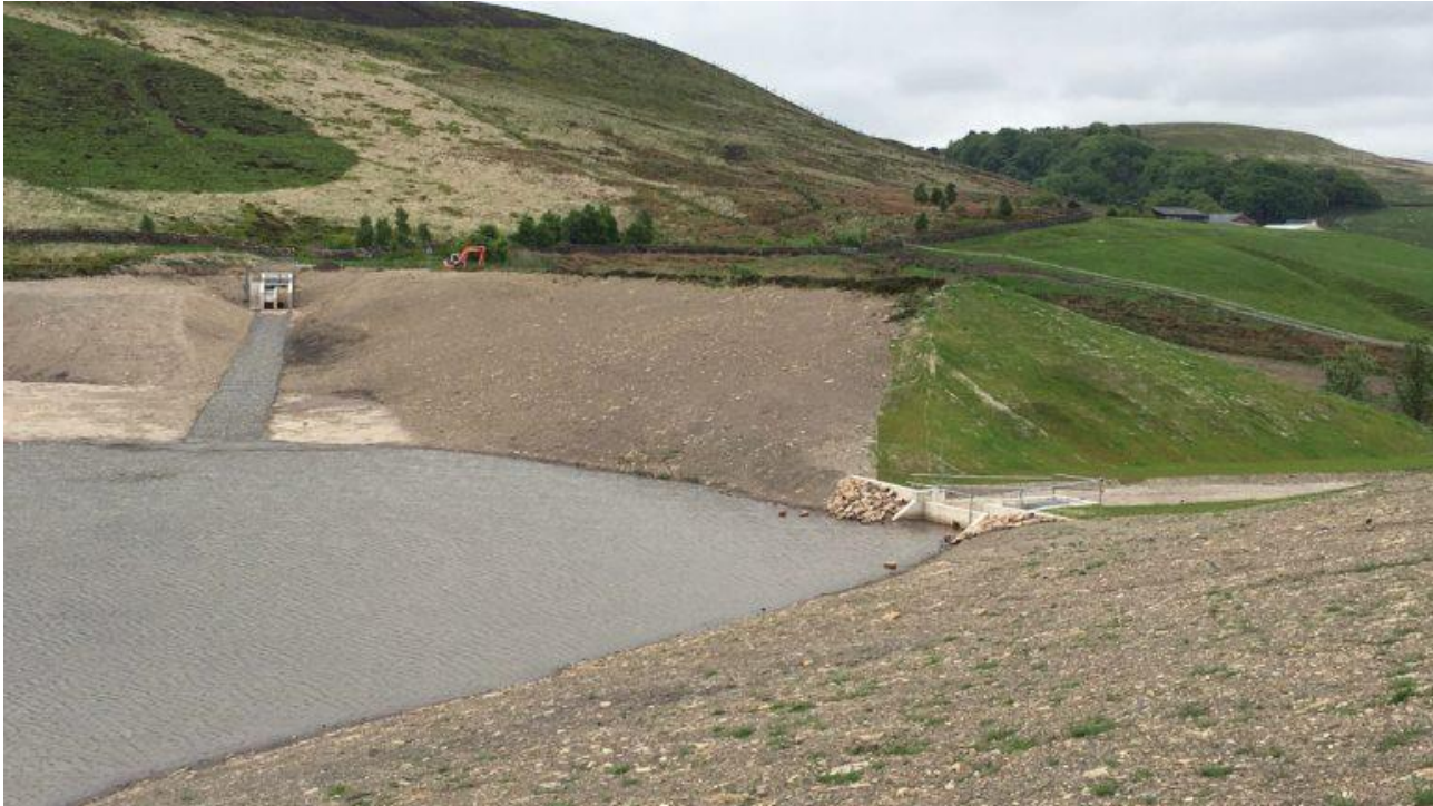
Figure 3 Sunnyhurst notch with overflow structure. The screening chamber can be seen at the top of the photograph
