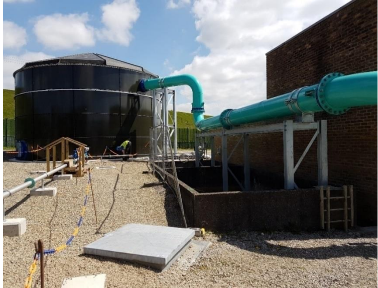
Figure 13: Installing start up to waste at all treatment works
