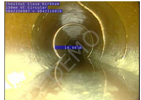
Figure 15: Build-up of silt, and circumferential cracking within a sewer
