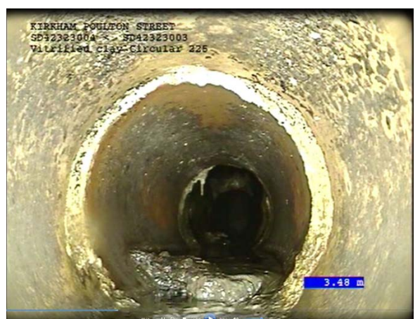
Figure 17: Partial blockage and protruding grout
