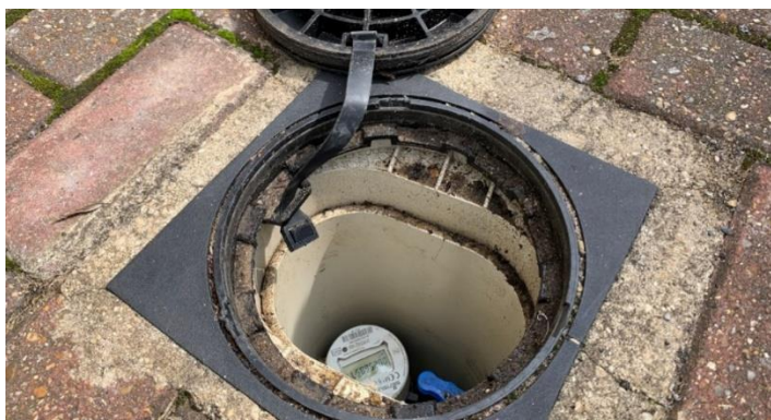
Water meter outside customer premise
