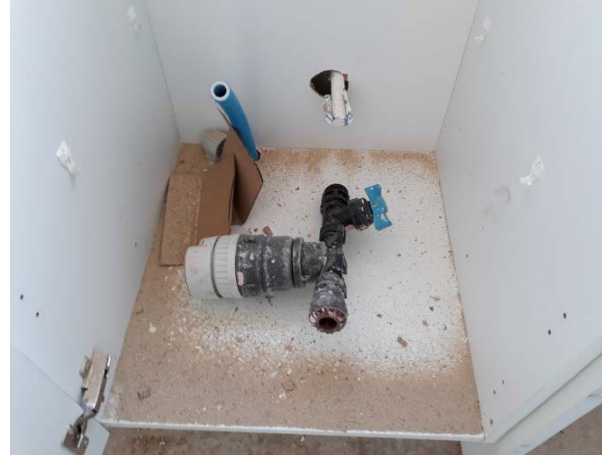
Internal meter install poor practice
