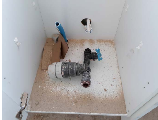
Internal meter install poor practice
