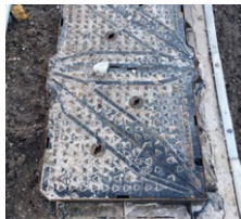
1200mm x 700mm chamber with isolation valves either side
