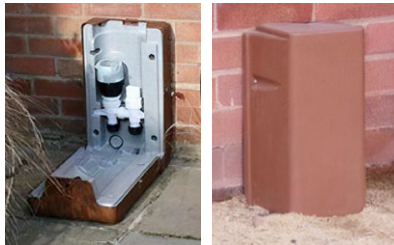
Wall mount box in situ and insu-duct
