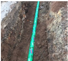
Spiral wrapped pipe with ID marker tape
