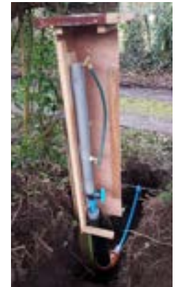
This is an example of a lockable box referenced in the spec drawing on the left.
