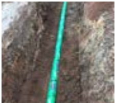
Spiral wrapped pipe with ID marker tape
