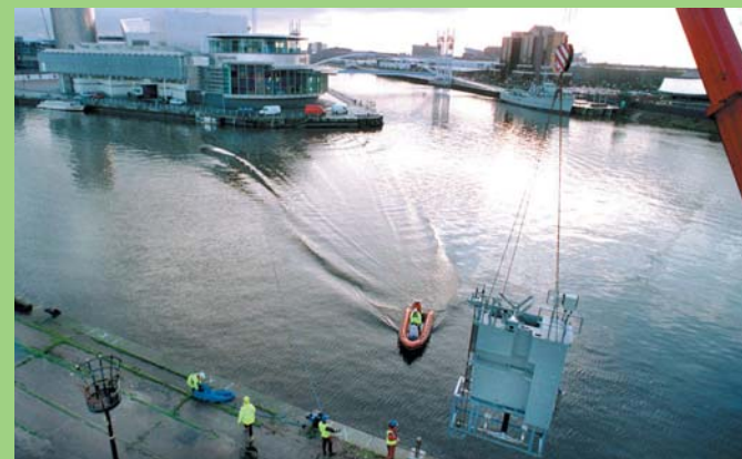
One of five oxygenation units being installed at Salford Quays, to breathe new life into the Manchester Ship Canal.
