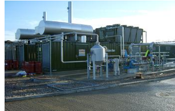
Combined heat & power installation
