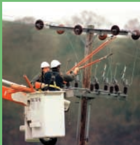
Live line or 'hot glove' working allows some operations to be performed on our 11kv network with the overhead wires live, so reducing the number of supply interruptions to our customers.
