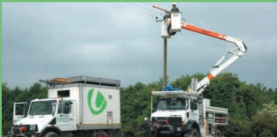
Live line or 'hot glove' working allows some operations to be performed on our 11kv network with the overhead wires live, so reducing the number of supply interruptions to our customers.
